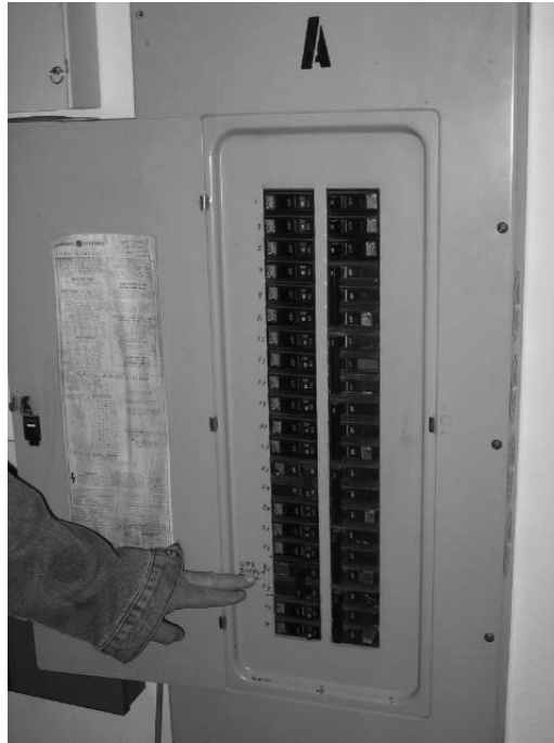
UPS AC Supply Breakers on panel A
