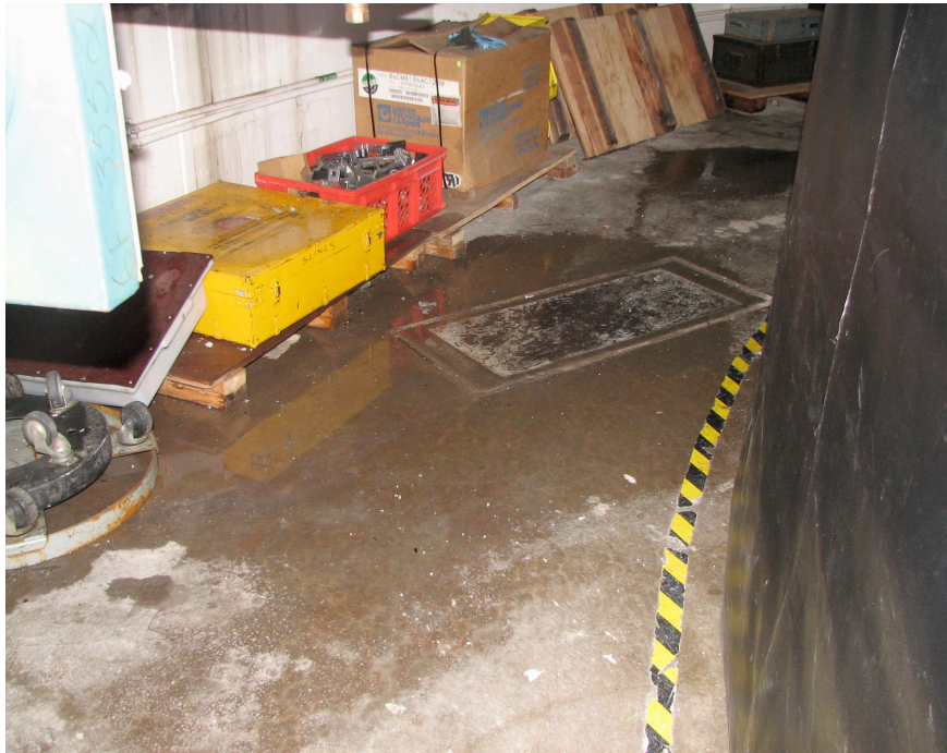
A puddle on the floor of the pit, where MAESTRO is to be stored.
