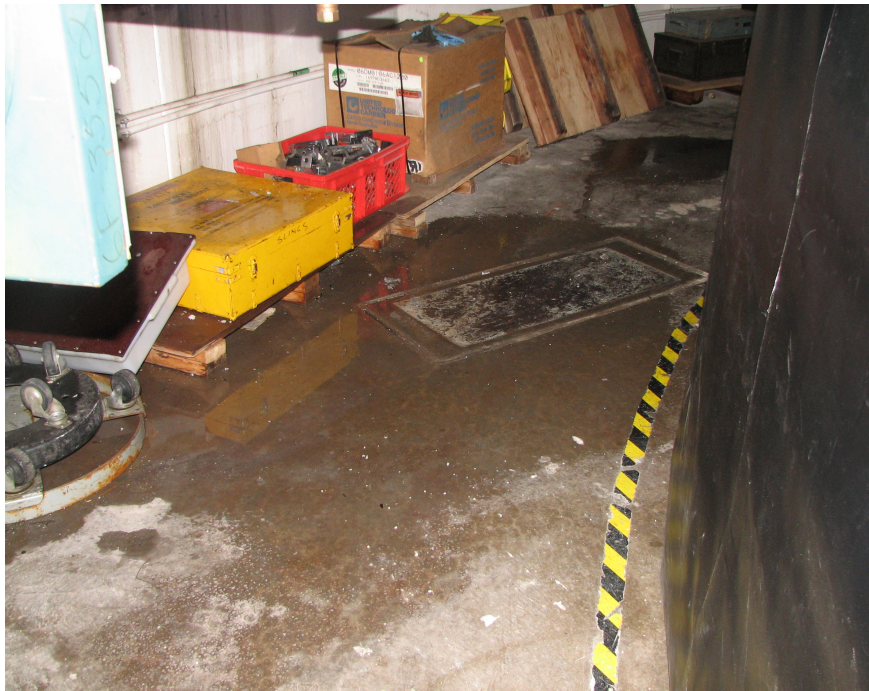
A puddle on the floor of the pit, where MAESTRO is to be stored.
